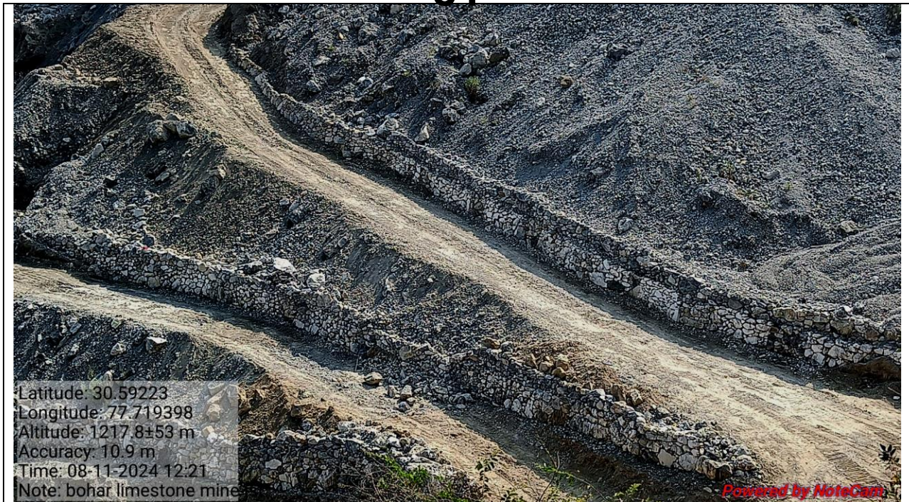
Photograph no. 5- Shows status of retaining wall structures provided at the slope of five benches in M/s Bohar lime stone mine
