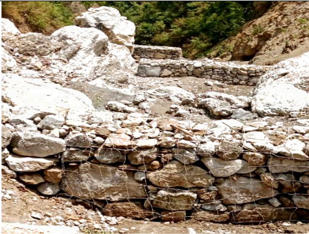
Photograph no. 6 – Shows status of retaining structures provided by M/s Bohar lime stone in the run off channel of seasonal dunga nallah to protect flow of debris and damage to property of local people
